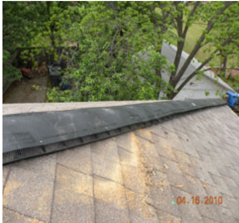
Vent installed on one of the four diagonal hips of the hip roof.
