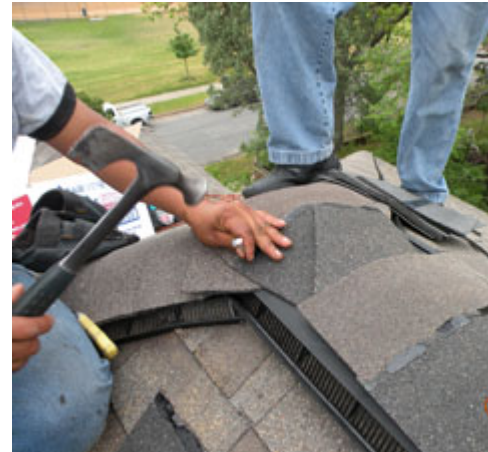
Cap shingles installed over the Hip Ridge Vent and ShingleVent II ridge vent intersection.
