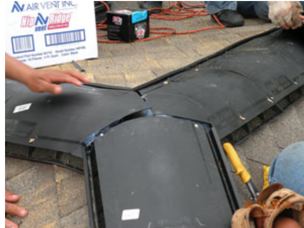
Hip Ridge Vent installed on two of the four diagonal ridges intersecting the horizontal ridge where ShingleVent II ridge vent is installed. Using tin snips or a utility knife, roofing contractors miter cut the Hip Ridge Vent to fit into ShingleVent II ridge vent.
